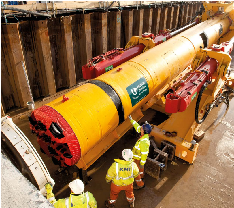
Equipment set-up at the launch pit: Pipe Thruster, Direct Pipe® machine, pipeline and control container.
