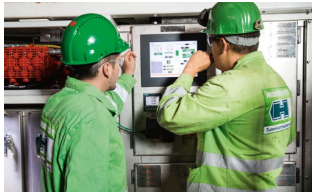
Power pack with PLC control and data recording system.
